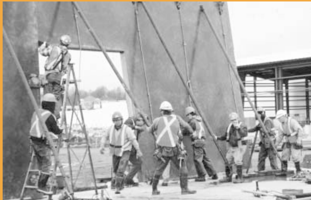
Carpenter crew places tilt-up wall for one of two buildings at the Vancouver City Works yard on Chess St. Smith Bros. Wilson superintendent Jim Morrison said there were only three typical panels in the entire job as the rest are one-off. "It's the first time we've ever done embossed panels," he said.
